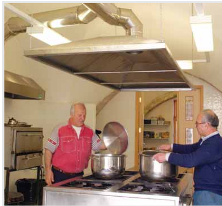
Tikkya Kitchen in the Industrial School- Dar Al Aytam Complex (after restoration )
