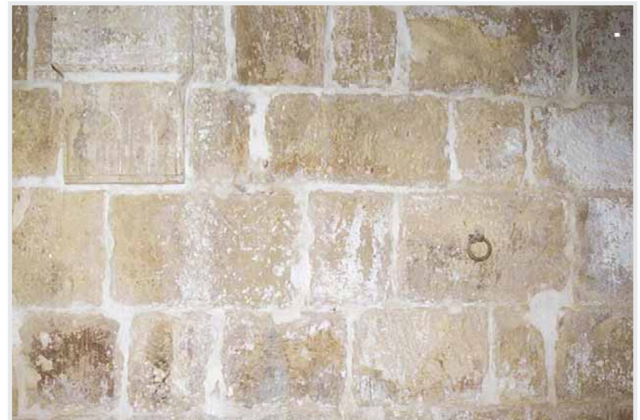
Pl.1.9 Springing of arches and in the main hall of Dar al-Sit Tunshuq al-Muzafariyya
